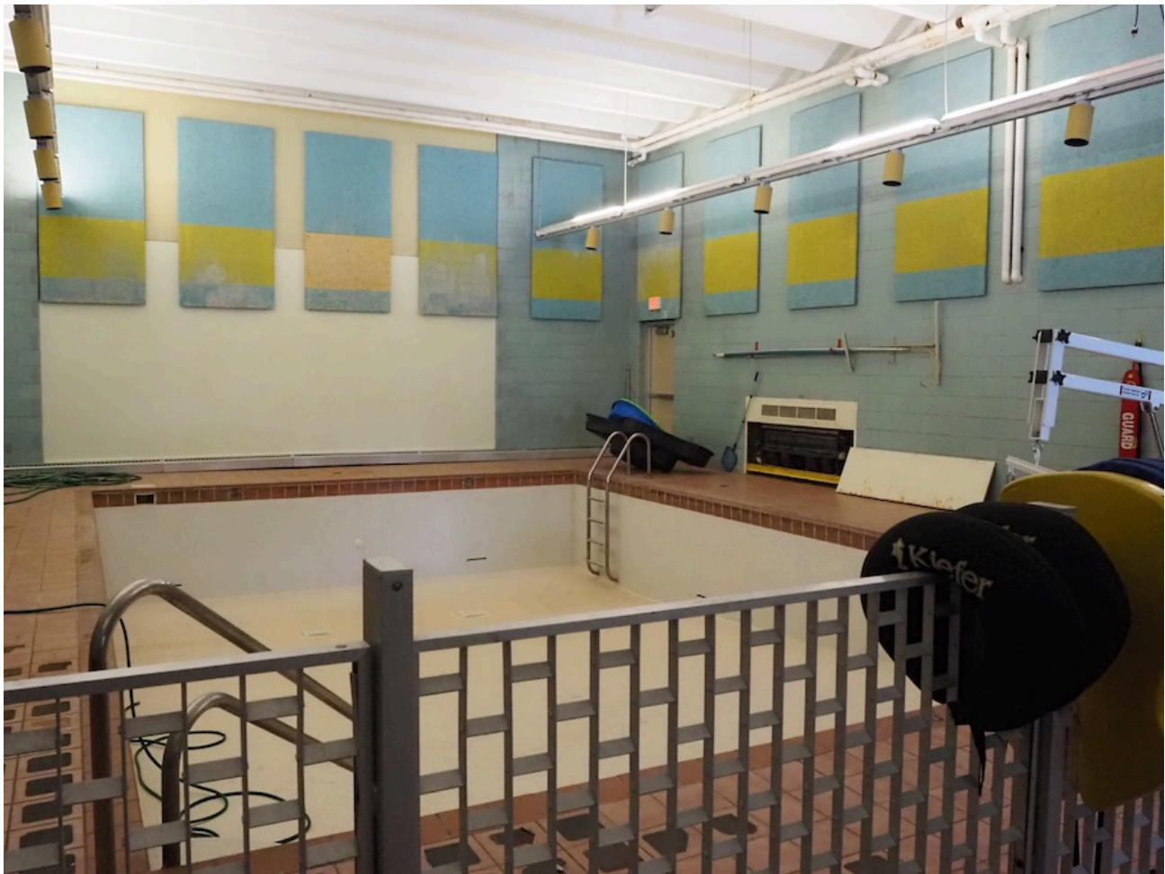
The pool at the Beekman Center in Lansing is in need of repairs and is not operational on Jan. 29, 2026. (Anna Liz Nichols for ELi)
